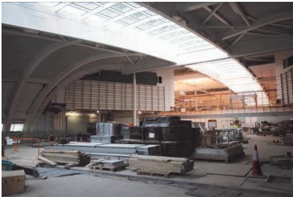
View of the land-side departures floor facing towards the centralised passenger security screening area. The linear fanlight in view stretches from the front to the back of the new terminal
